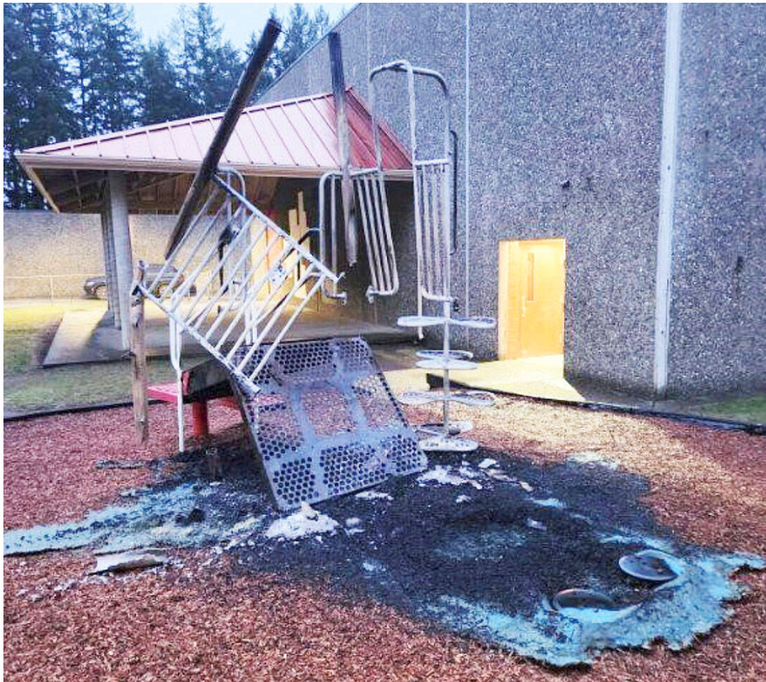
SKSD courtesy photo The remains of a preschool playground structure at Burley Glenwood Elementary.
